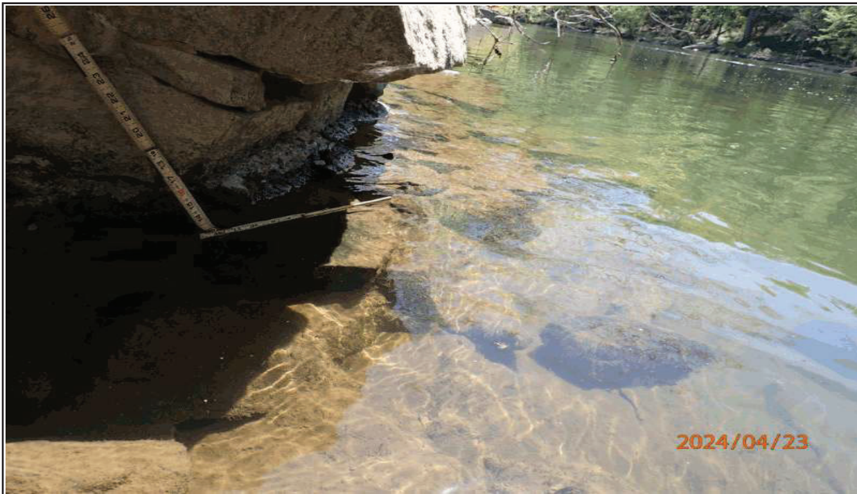
34 NORTH MASONRY ABUTMENT, EAST THRUST BLOCK, VOID IN REPOINTED SECTION
