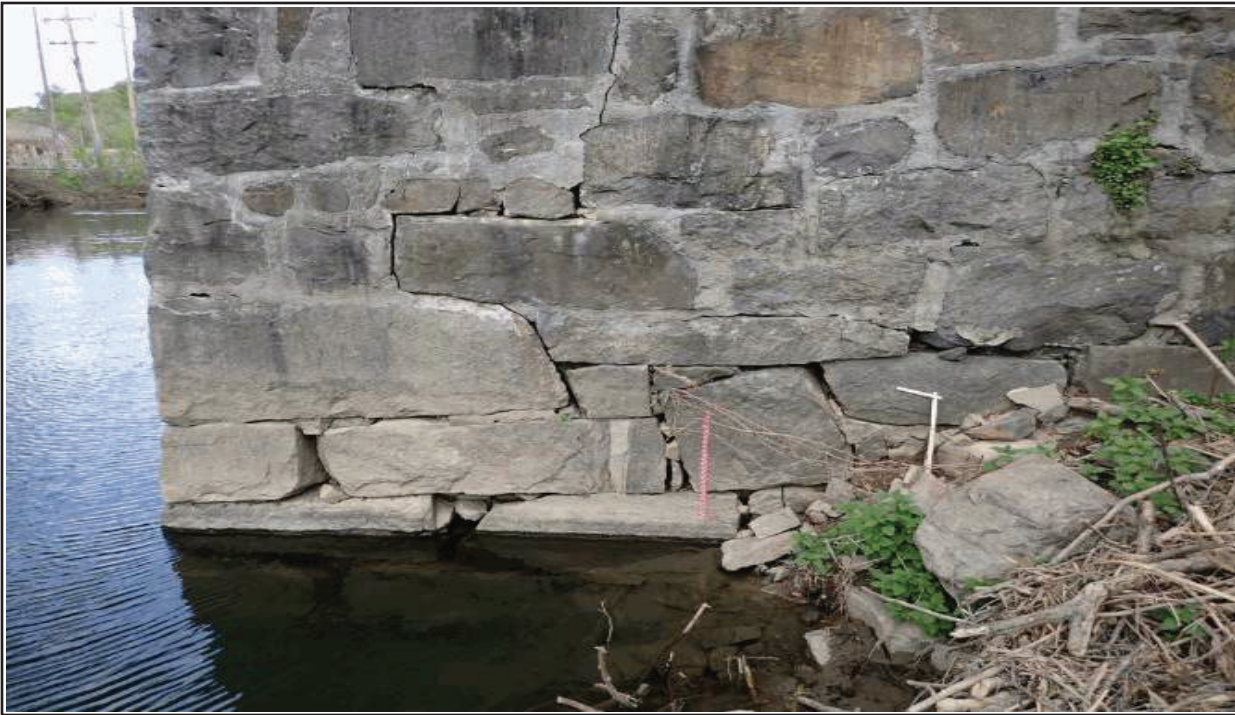
35 SOUTHWEST MASONRY WINGWALL - AREA OF MISSING MORTAR AND DISPLACED STONES
