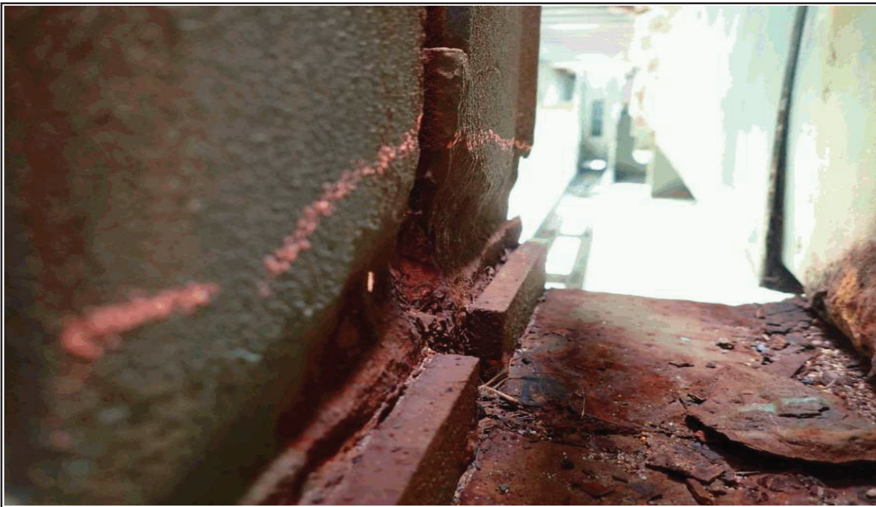
22 EAST TRUSS, L5-U5 INBOARD ANGLE LEGS ABOVE L5, WEST FACE - SECTION LOSS WITH ACTIVE CORROSION
