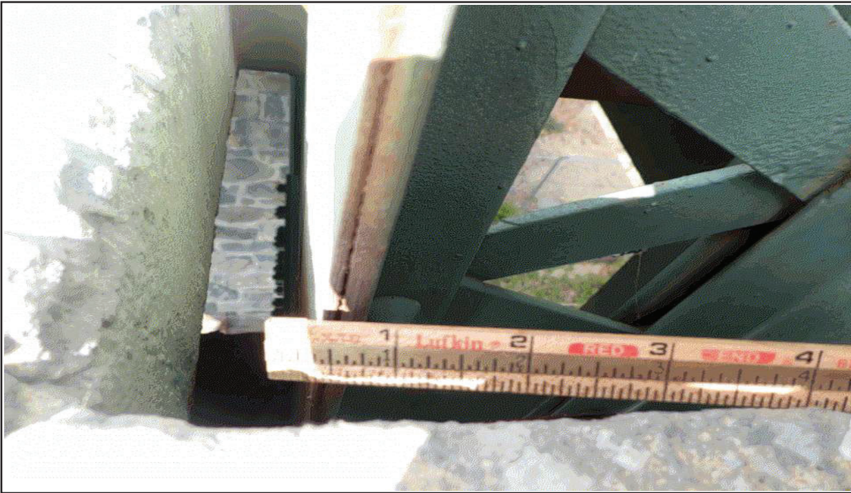
21 EAST TRUSS, L5-U5, SOUTHWEST ANGLE EDGE - PACK RUST CAUSING SEPARATION
