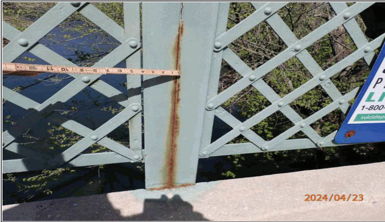
9 WEST RAILING, NORTH END - TYPICAL PACK RUST BETWEEN POST ANGLES
