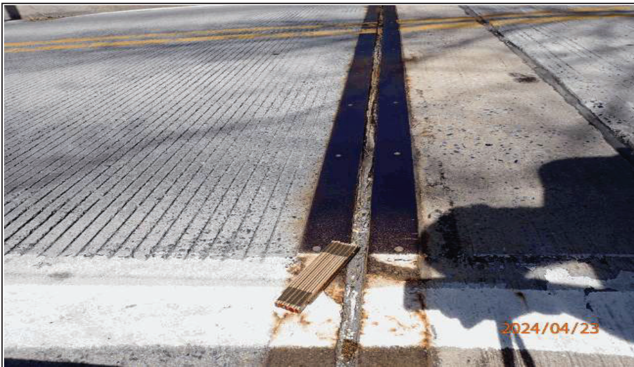
12 NORTH COMPRESSION JOINT SEAL - FULLY DEBONDED & FILLED WITH DEBRIS
