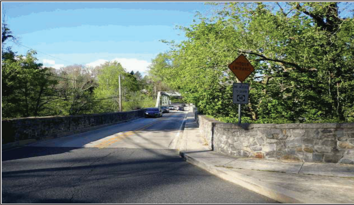
37 SOUTH APPROACH - VERTICAL CLEARANCE & LOAD POSTING NOT VISIBLE DUE TO VEGETATION
