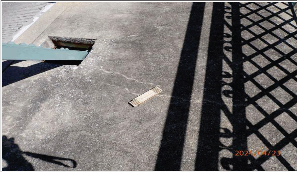
11 EAST SIDEWALK, NEAR MIDSPAN - FULL-WIDTH HAIRLINE CRACK WITH EFFLORESCENCE
