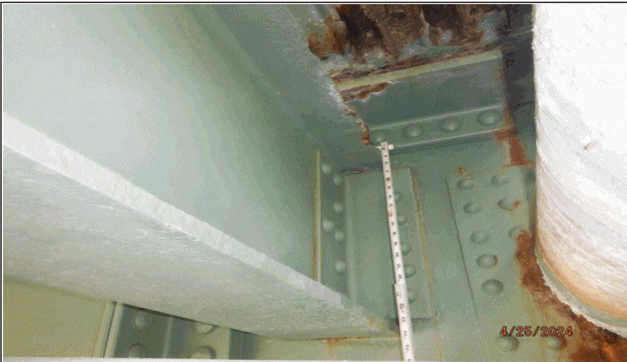
30 PANEL 1, STRINGER 1, EAST TOP FLANGE NEAR FLOORBEAM 1 CONNECTION - KNIFE EDGING AND PAINTED OVER PITTING
