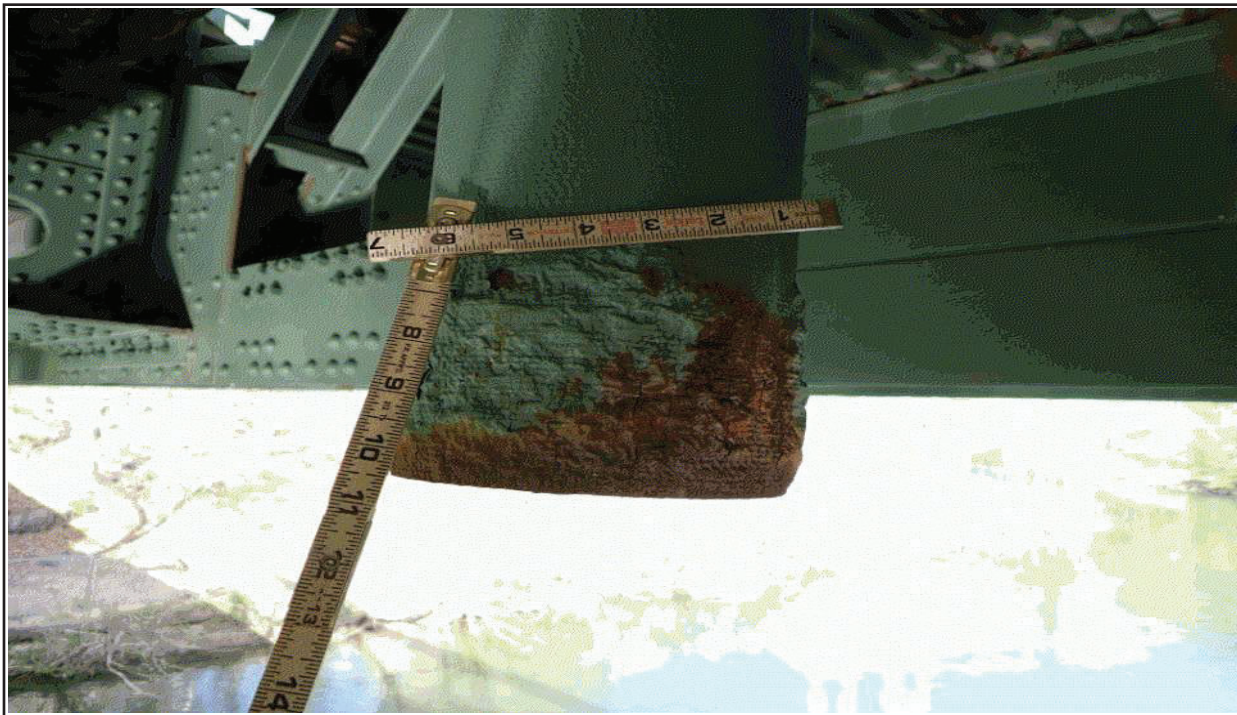
14 EAST DRAIN OUTLET, BETWEEN FLOORBEAM 1 & 2 - CORROSION WITH SECTION LOSS
