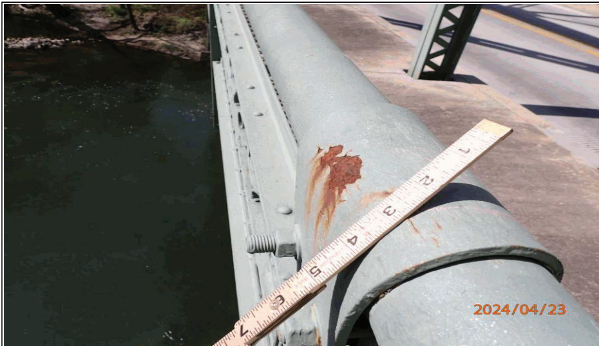
10 EAST RAILING, 2ND POST FROM NORTH END - TYPICAL ACTIVE CORROSION
