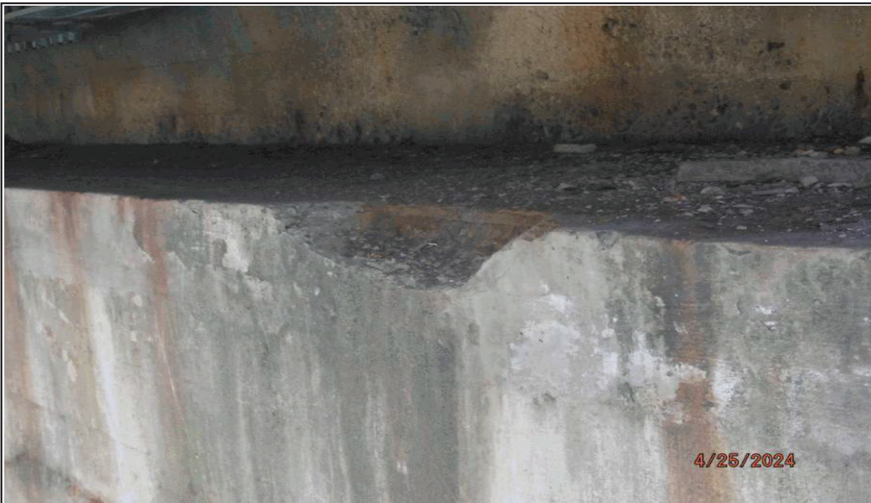
32 SOUTH CONCRETE ABUTMENT, BELOW STRINGER 1 - EDGE SPALL
