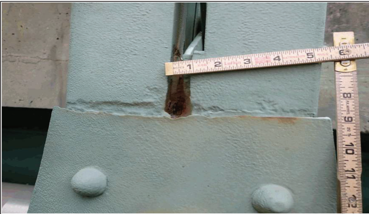
20 WEST TRUSS, L5-U5, EXTERIOR FACE OF OUTBOARD ANGLE @ L5 CONNECTION - PAINTED OVER SECTION LOSS
