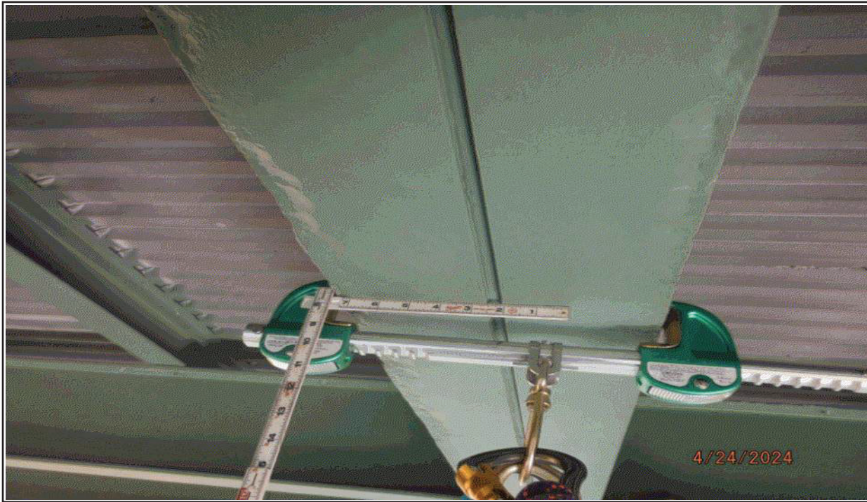
27 FLOORBEAM 3, WEST END, NORTH AND SOUTH BOTTOM FLANGE ANGLES - SECTION LOSS
