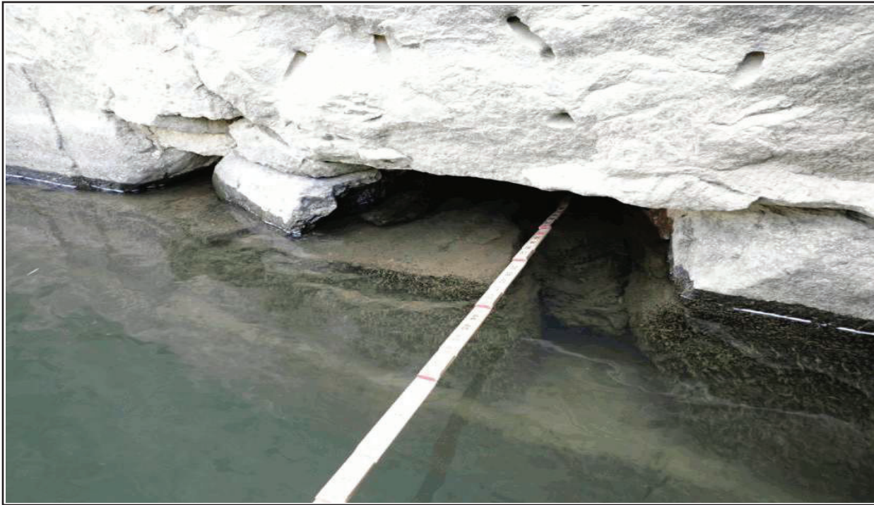
33 SOUTH MASONRY ABUTMENT, NEAR WEST END - AREA OF MISSING STONES
