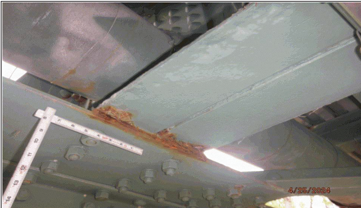
28 FLOORBEAM 5, WEST END, CONNECTION TO LATERAL GUSSET PLATE - SECTION LOSS WITH ACTIVE CORROSION
