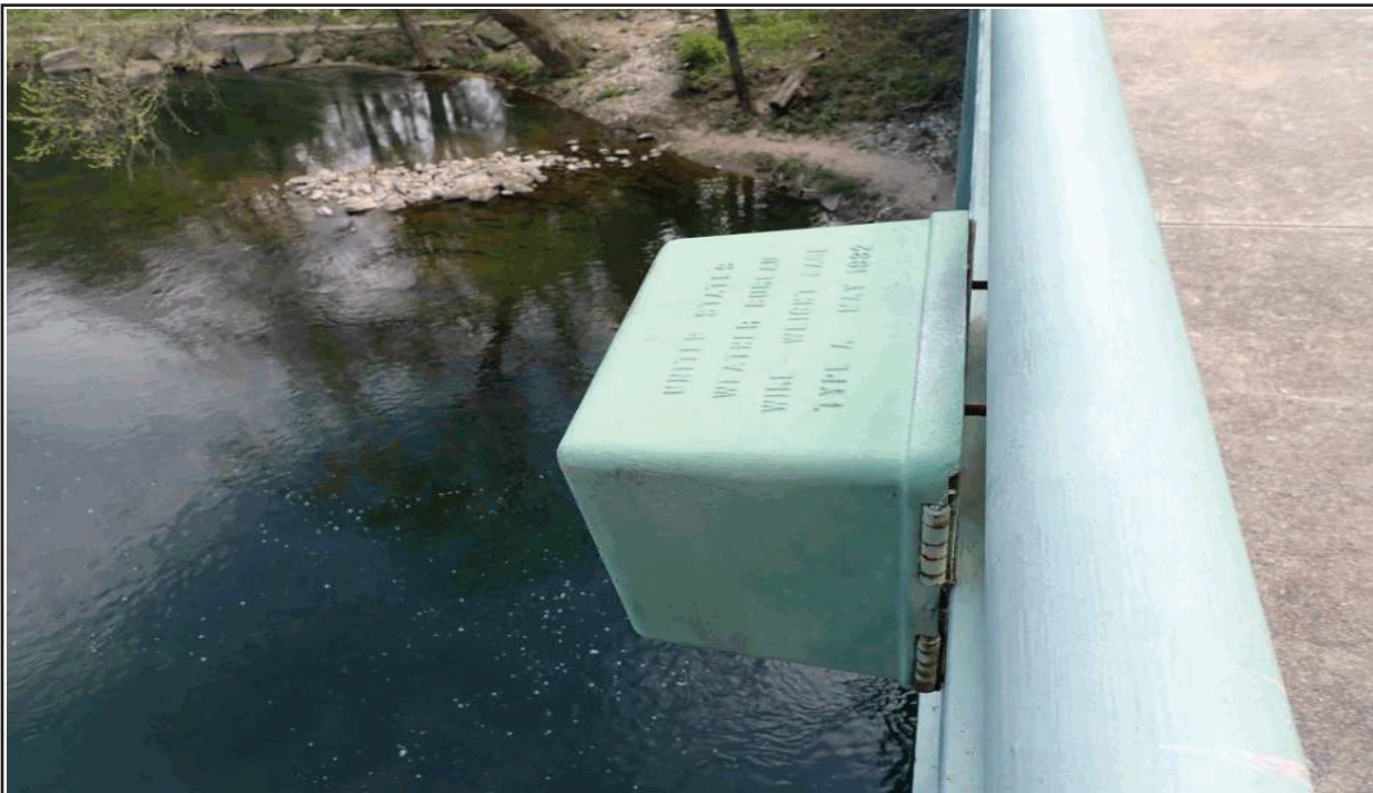
36 EAST RAIL, MIDSPAN - STREAM GAUGE ATTACHMENT
