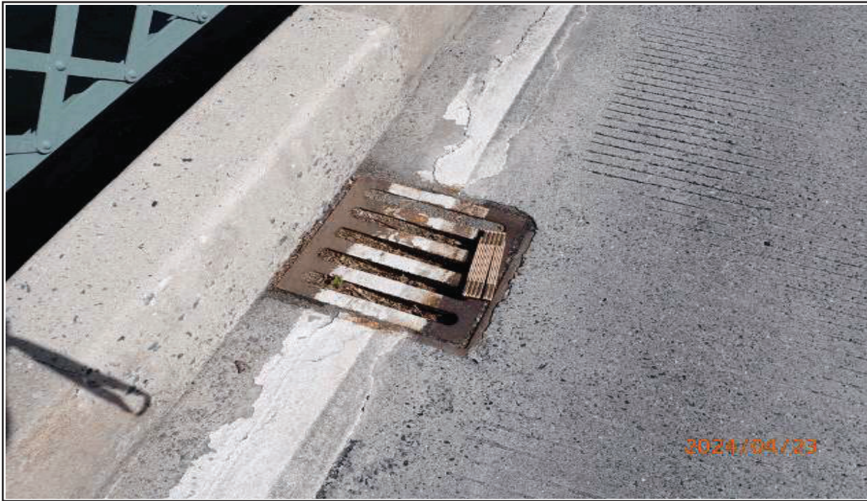
13 SOUTHWESTMOST DRAIN - TYPICAL CLOGGED SOUTH DRAIN
