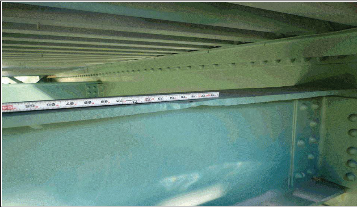
31 PANEL 3, STRINGER 1, WEST TOP FLANGE NEAR FLOORBEAM 2 - SECTION LOSS
