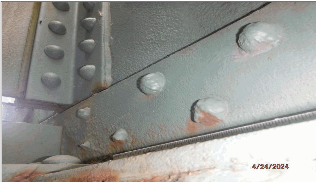
24 WEST TRUSS, L4 OUTBOARD GUSSET, INTERIOR CONNECTION - RIVET HEADS WITH SECTION LOSS
