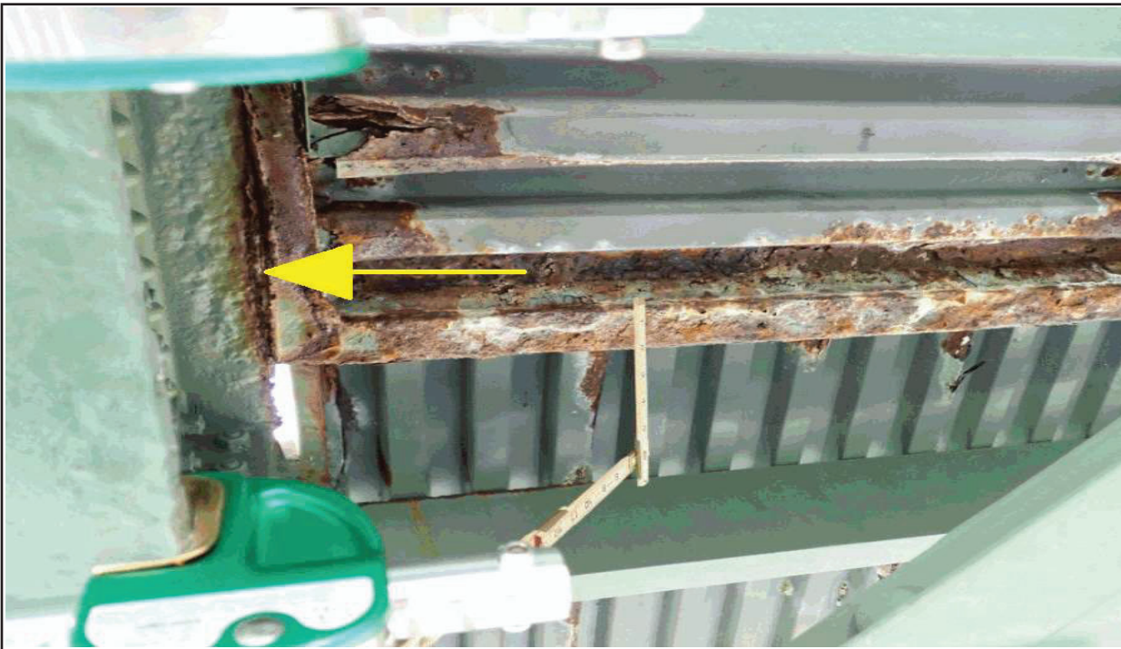
26 FLOORBEAM 1, EAST SIDE, UNDERSIDE OF TOP FLANGE - SECTION LOSS
