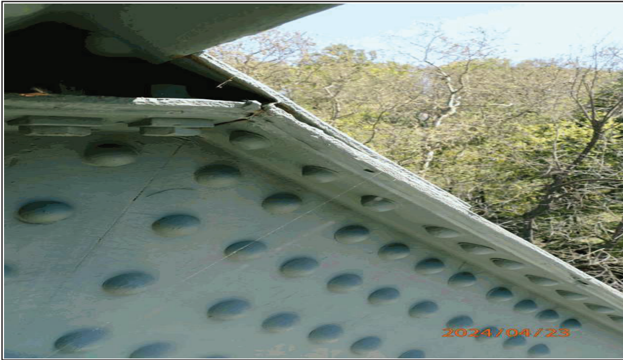
15 SOUTH PORTAL, CONNECTION PLATE TO U1E, WEST EDGE - PAINTED OVER SECTION LOSS & PACK RUST
