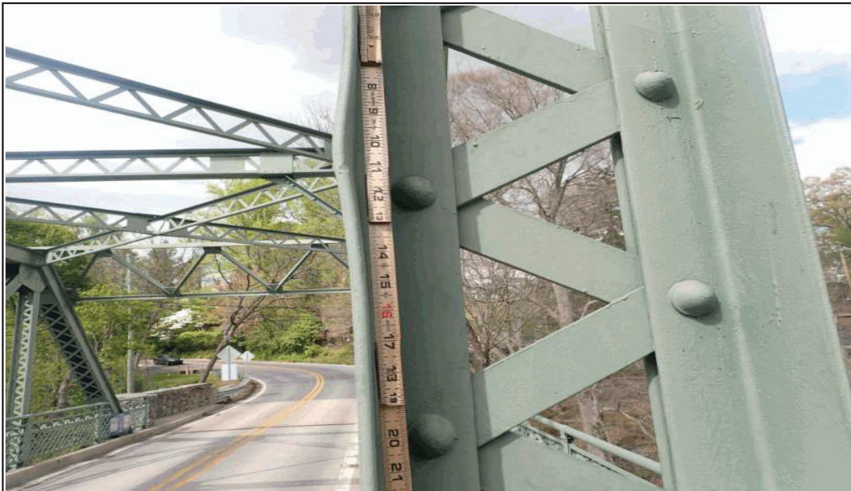
18 EAST CHORD, L3-U3, SW ANGLE, MID-HEIGHT - DEFORMATION IN FLANGE
