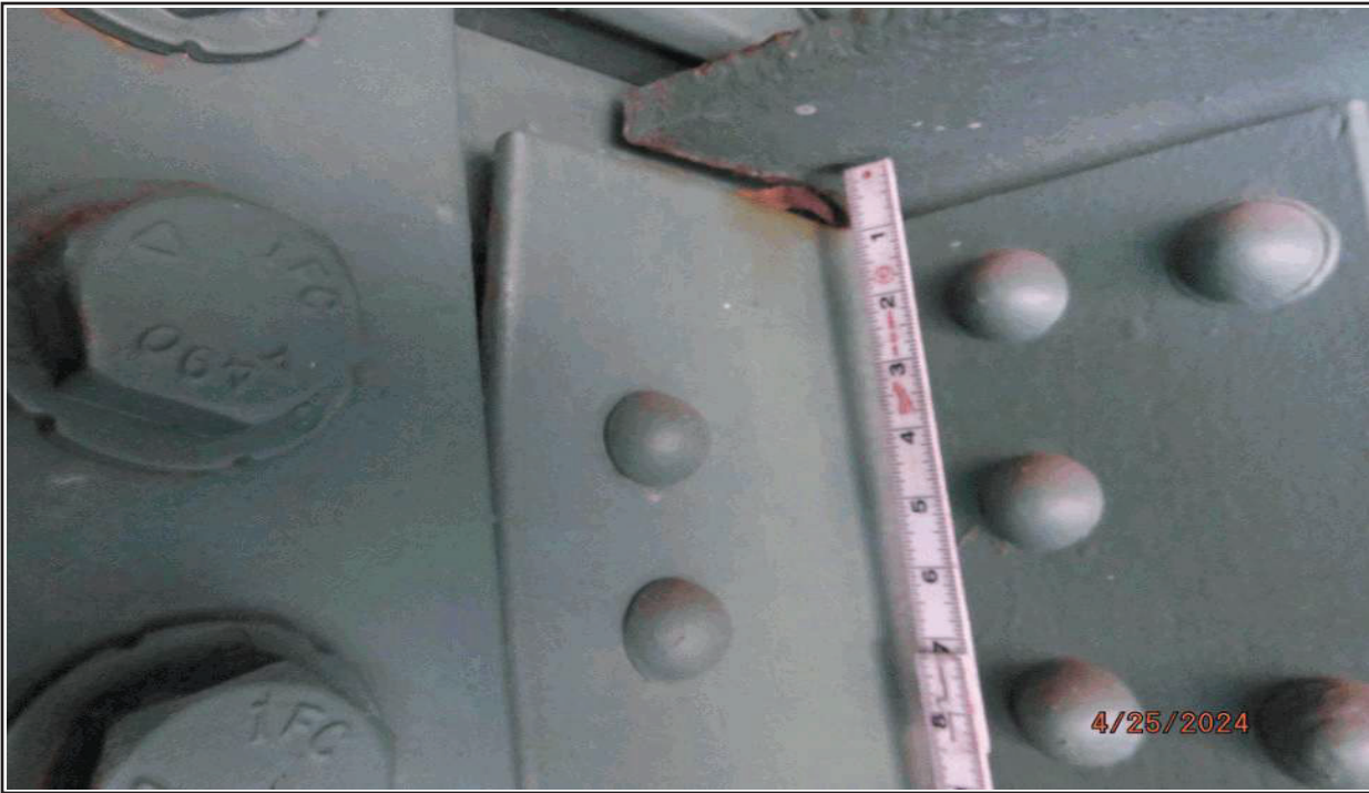
29 PANEL 1, STRINGER 1, WEST CONNECTION ANGLE TO FLOORBEAM 0 - ANGLE NOT FLUSH
