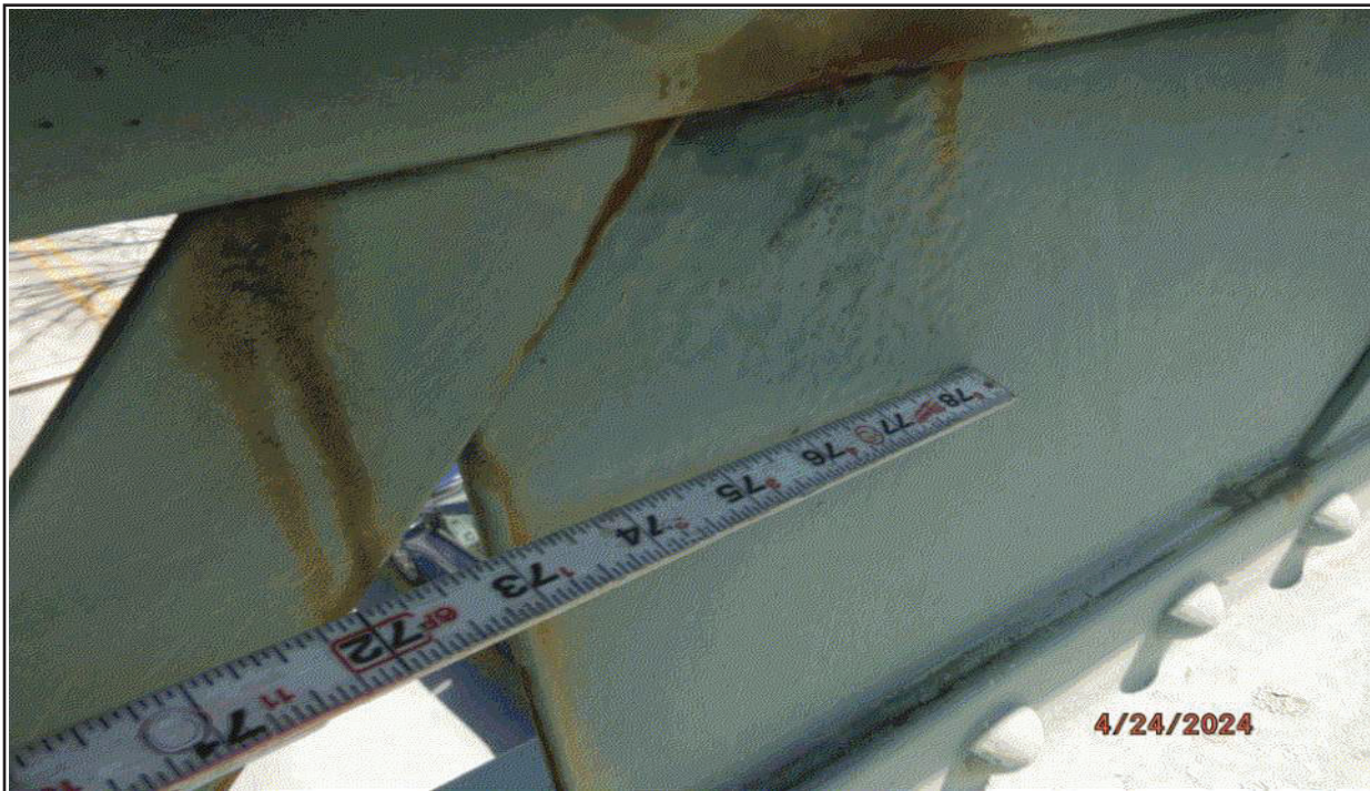
16 BATTEN PLATES ADJACENT TO U4W & U4E, NORTH FACE - AREAS OF PITTING
