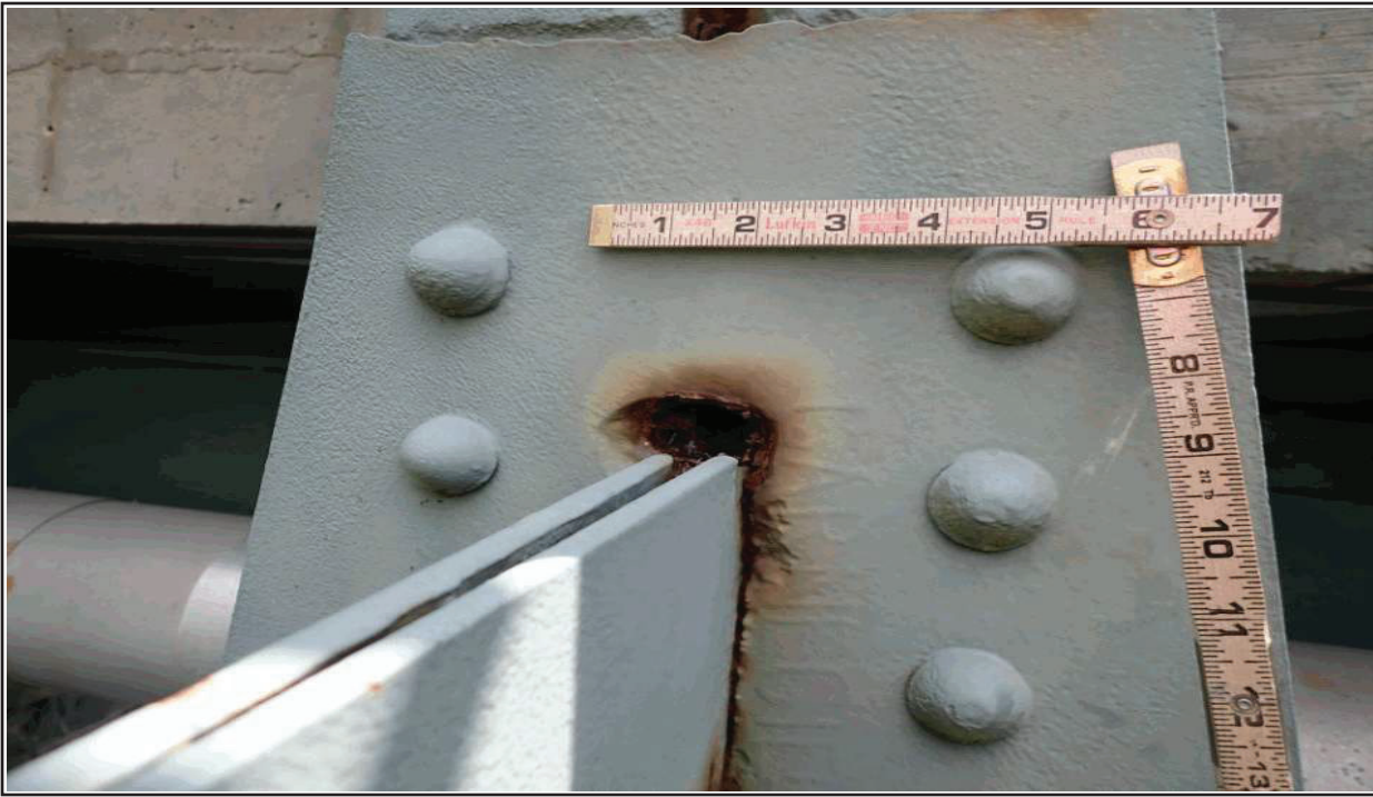
25 WEST TRUSS, L5 OUTBOARD GUSSET PLATE AND STRAPPING PLATE CONNECTION - SECTION LOSS
