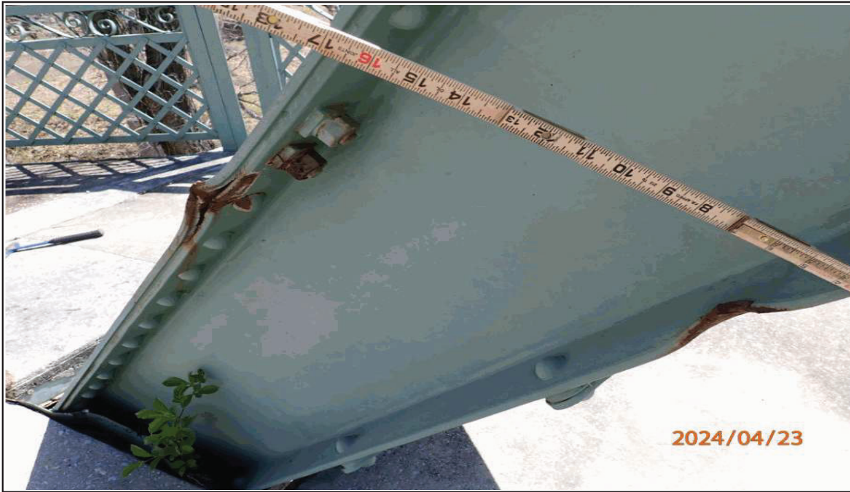
17 EAST CHORD, U5-L6, NORTHEAST CORNER - IMPACT DAMAGE WITH CORROSION
